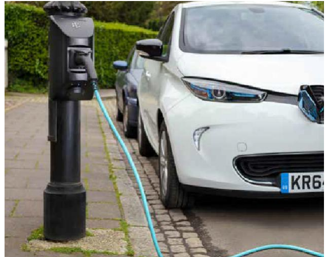
Figure 79: Example of on-street electric vehicle charging points.
