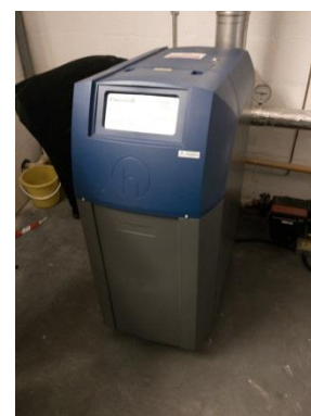
Figure 28: Purewell gas boiler
