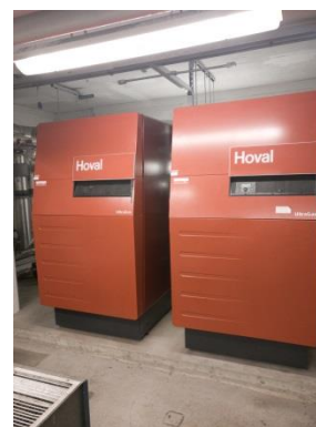
Figure 31: Parklands 350kW gas boilers
