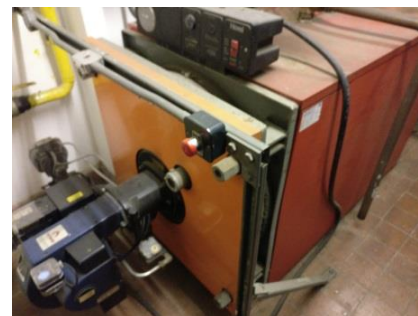
Figure 27: Centre management suite boilers
