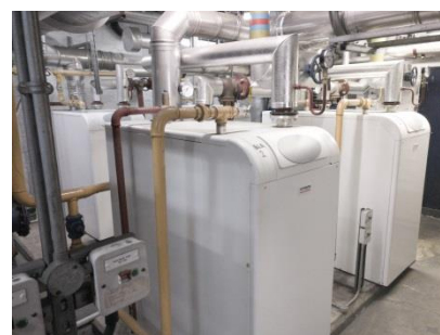
Figure 32: Anvil gas boilers
