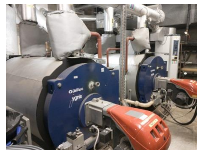
Figure 29: Deanes 520kW gas boilers
