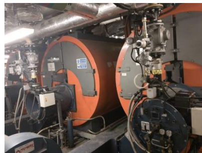
Figure 23: Hospital LTHW gas boilers
