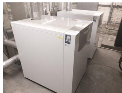
Figure 30: Goldings 80kW gas boilers
