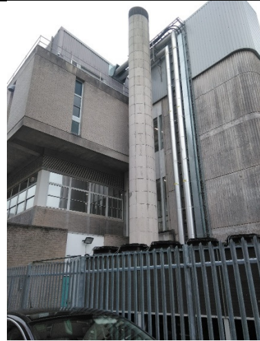
Figure 6 Main hospital flue for the main plant room boilers
