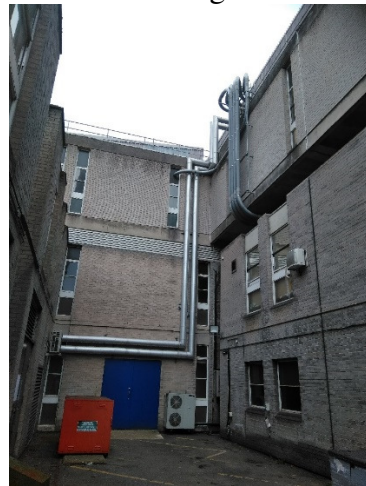
Figure 7 Image taken from the entrance to the plant room onto the courtyard outside
