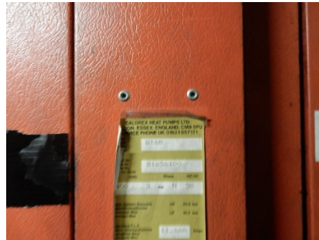
Figure 23 the swimming pool top up boiler that backups the air handling units is used to heat the pool water
