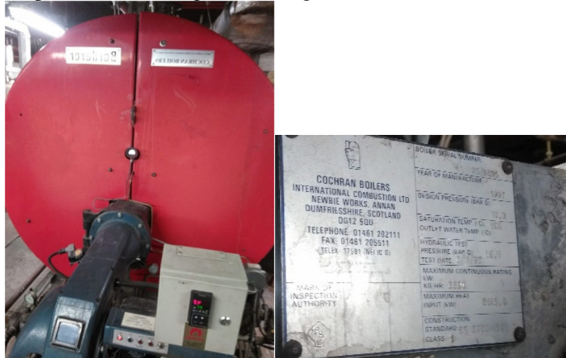
Figure 5 one of the 2 Cochran steam boilers and its plate
