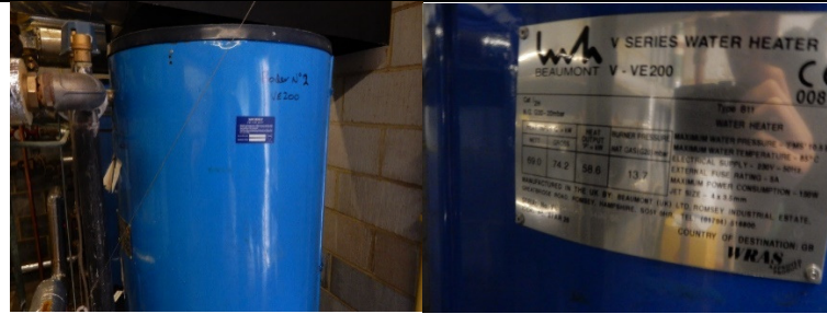
Figure 22 The hot water heaters used in the domestic hot water plant room
