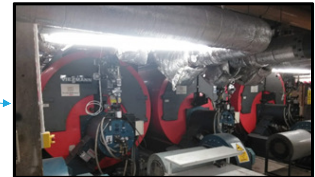
Figure 2.1.4 ECC – existing hospital plantroom (main building)
