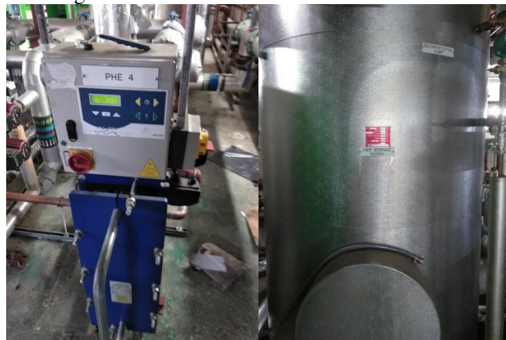
Figure 2 one of the heat exchanges (left) and 4000litre HWS storage vessel (right).
