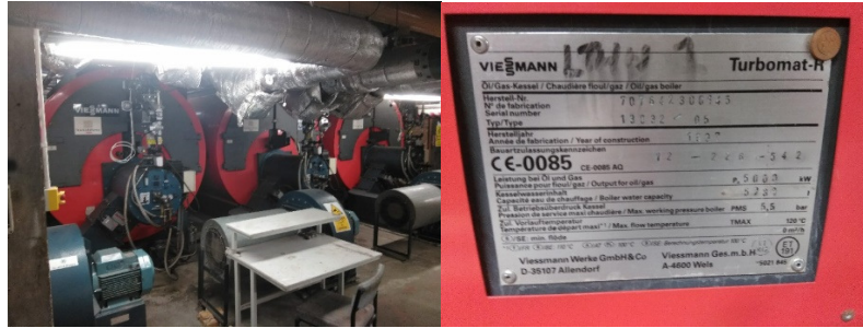
Figure 4 5MW LTHW Viessmann boilers
