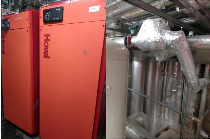
Figure 16 two Hoval calorifiers (left) and the manifold for the central heating (right)
