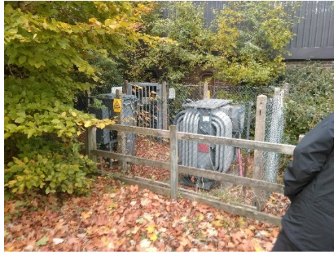
Figure 12 The substation next to the laundry
