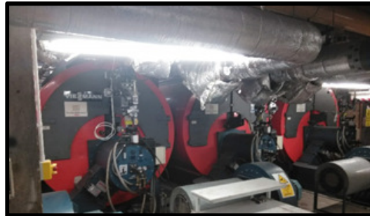
Figure 1.4.1 Hospital LTHW boilers
