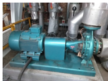
Figure 3 Heat network shunt pump
