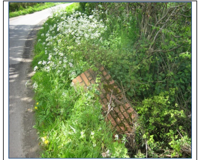
Picture 11 Possible reason for previous upstream flooding! Bridge abutment on Folly Lane blocking part of the Watercourse
