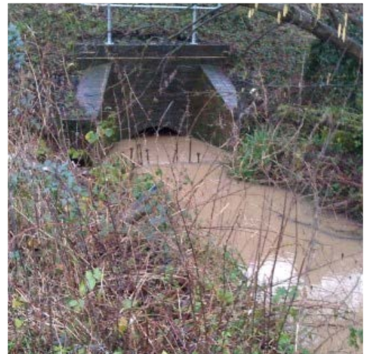
Picture 5 Stream north of Oakmead and Clift Meadow barely able to flow under the railway. Debris from the badly maintained hedge/stream could easily reduce the capacity of this culvert. This culvert takes the run-off from about 34 Hectares of agricultural land, the football pitch and Clift Meadow. It also handles the highway drainage from numerous small housing developments off the Street.
