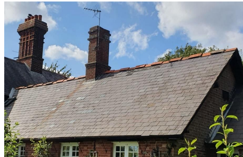
Figure 52. Laundry Cottage, 45 Home Farm Lane. Rear single storey wing with 'steam' ridge tiles. Notable Structure.
