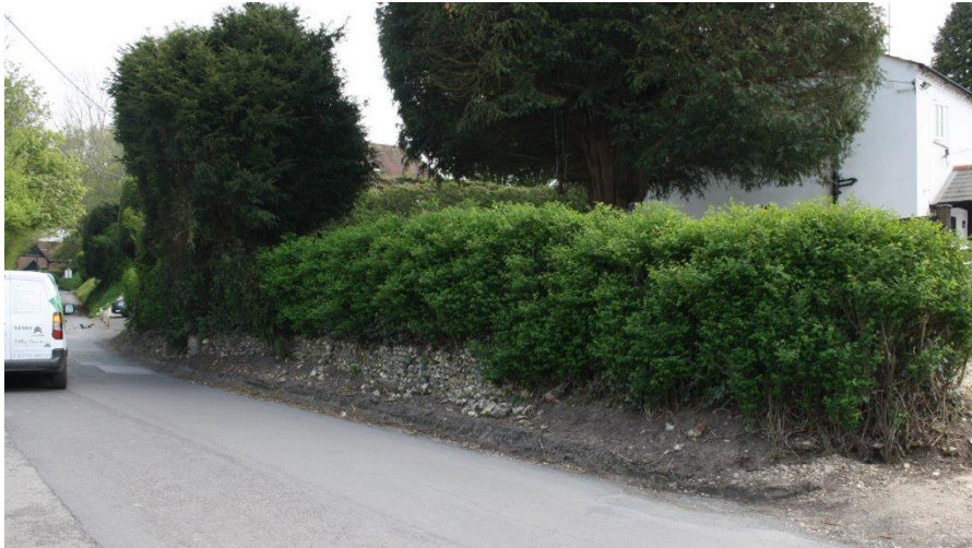
Figure 42: Flint bank to south of vehicle entrance at Cuckoo Bushes, Popham Lane. Notable Structure.
