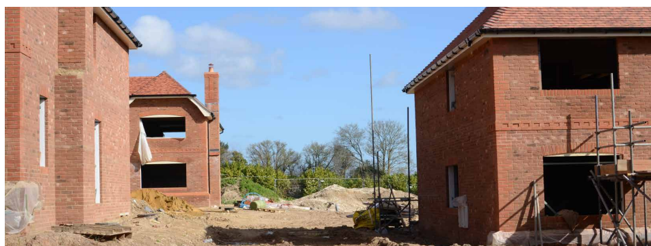
This new development on Woods Lane is an example of backland development that has eroded the linear 'one-plot-deep' character of the Plan Area
