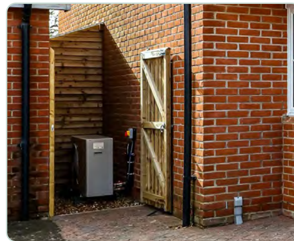
Figure 71: Example of a visually screened heating pump appropriate to the context of the building vernacular. Image credit: Daikin, Source: https://www.idealhome.co.uk
