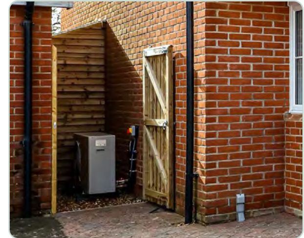
Figure 71: Example of a visually screened heating pump appropriate to the context of the building vernacular. Image credit: Daikin, Source: https://www.idealhome.co.uk
