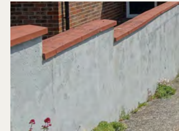
Smooth concrete or cement wall with little detailing
