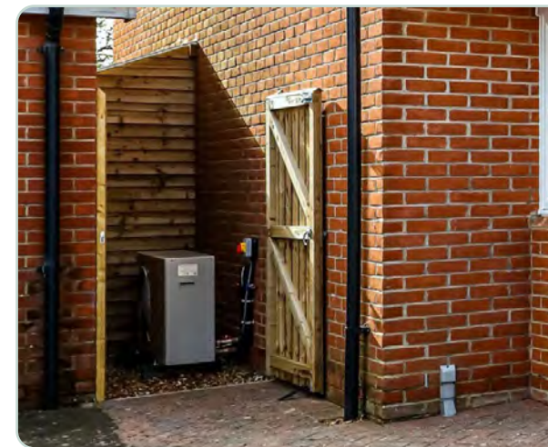
Figure 71: Example of a visually screened heating pump appropriate to the context of the building vernacular. Image credit: Daikin, Source: https://www.idealhome.co.uk
